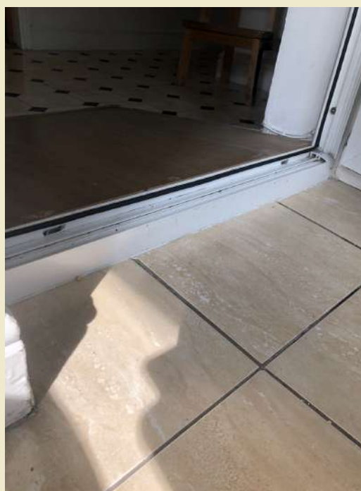
Photo 4: Dining room doorway, a trip hazard
